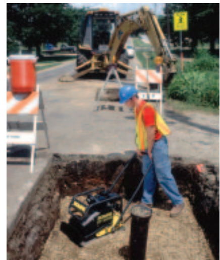
BP 25/48 in operation
